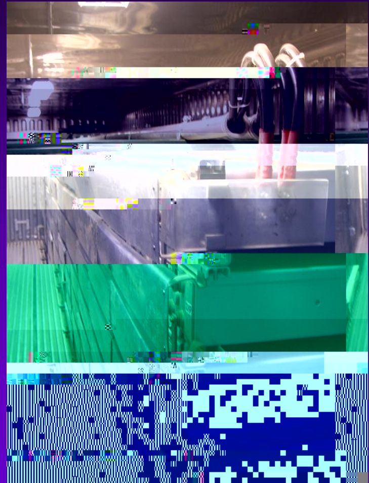
Batteries 3MW Total
